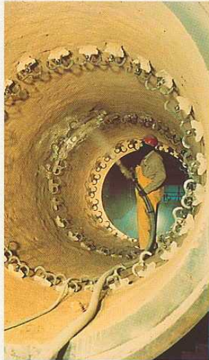
Cement Kiln - Chain Section, South Africa
